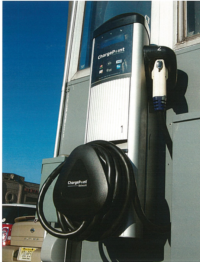
Electric car charging station in Newark, Essex County.
