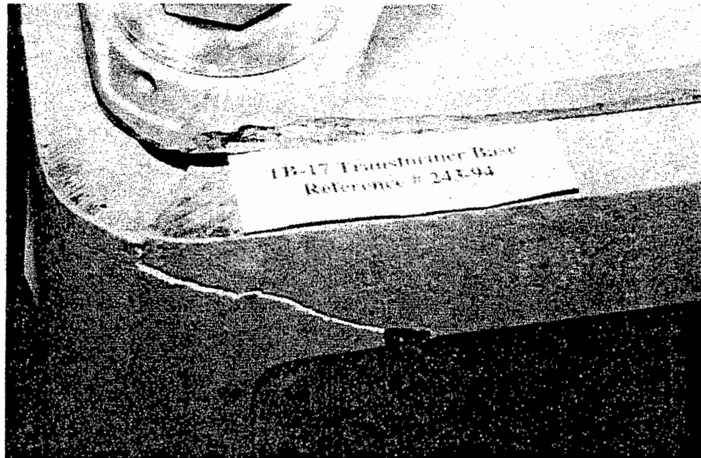
Figure 3-2 Cracked Transformer Base where Shoe Base Bolts on.
