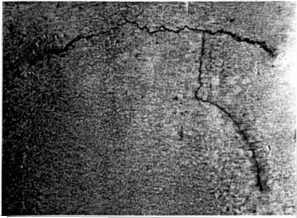
Figure 3-14 Fatigue Crack in Wall of Transformer Base of Specimen S-6
