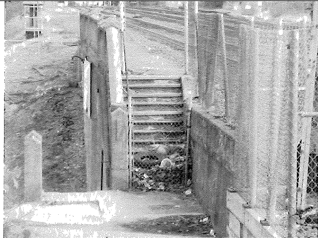
9. TRASH ON STAIRCASE @ CHURCH PL & NO GROVE ST
