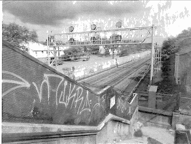
19. GRAFFITI ON STAIRCASE AT CHURCH PL FOOT BRIDGE
