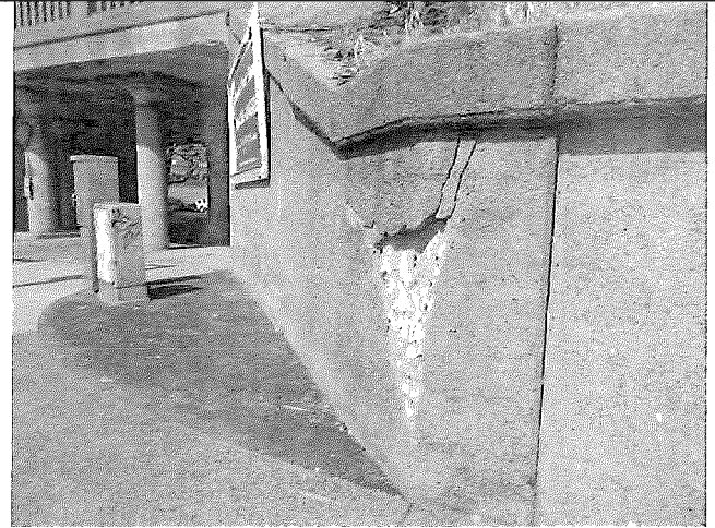
8. CRACK IN WALL AT FREEWAY DR EAST & SO BURNET
