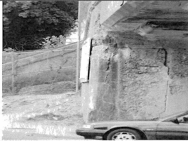
22. SPLALDING & CRACKS @ SPRINGDALE AVE UNDERPASS
