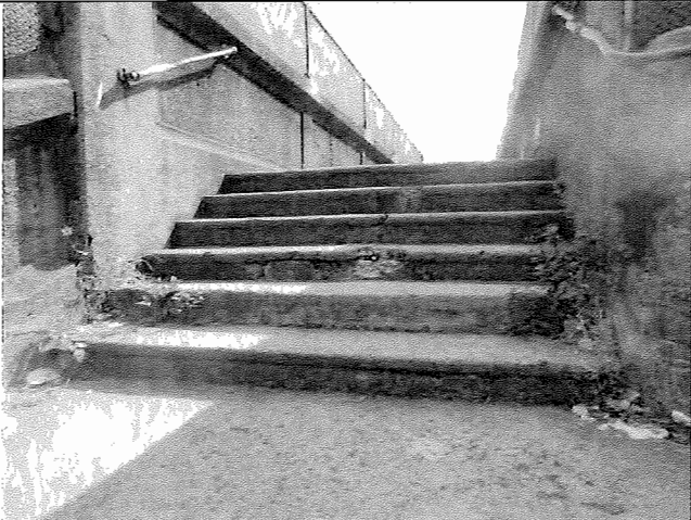
17. CHIPPED STAIR ON FOOT BRIDGE AT CHURCH PL & NO MAPLE AVE
