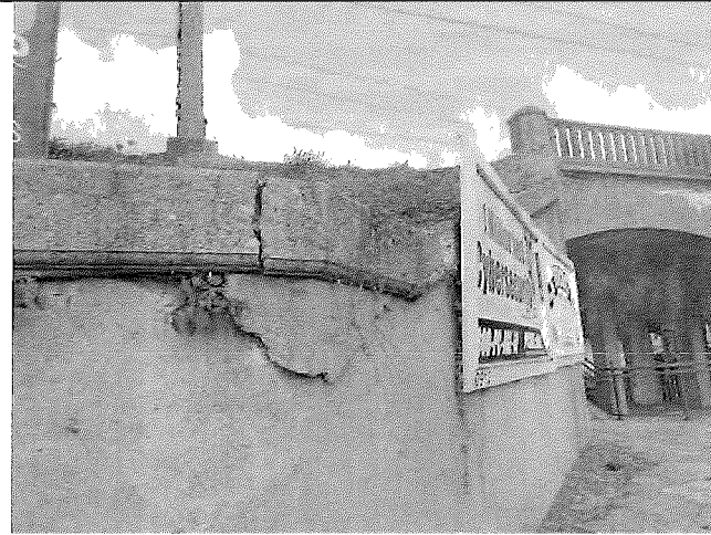
7. CRACKS IN WALL @ FREEWAY DRIVE EAST & MLK BLVD
