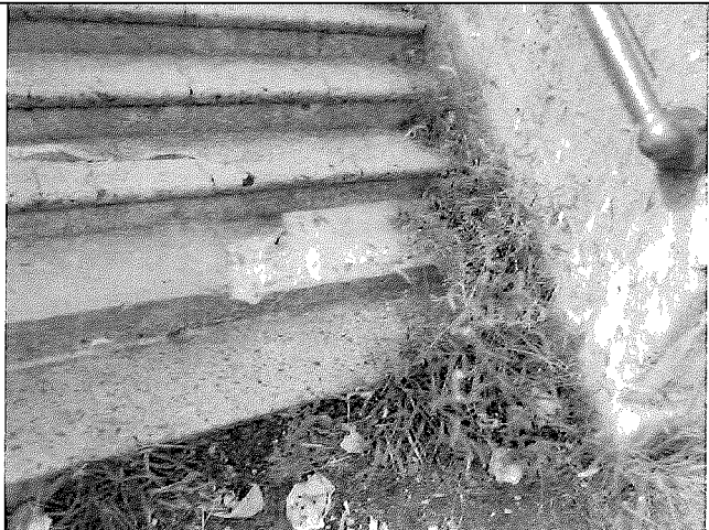
11. CHIPPED STEP AT CHURCH PL & NO MAPLE AVE
