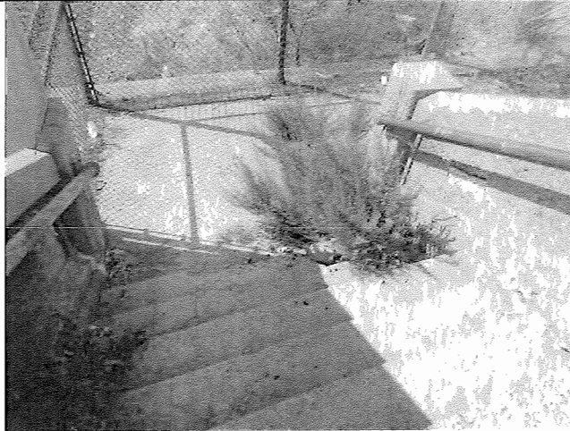
13. OVERGROWN WEEDS AT FOOT BRIDGE CHURCH PL & NO. MAPLE AVE
