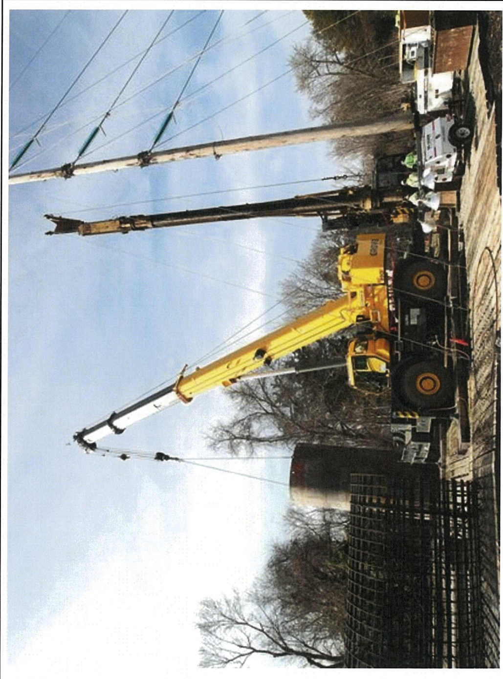
Oceanview Transmission project construction in Neptune. (Photo: Courtesy: Jersey Central Power & Light)
