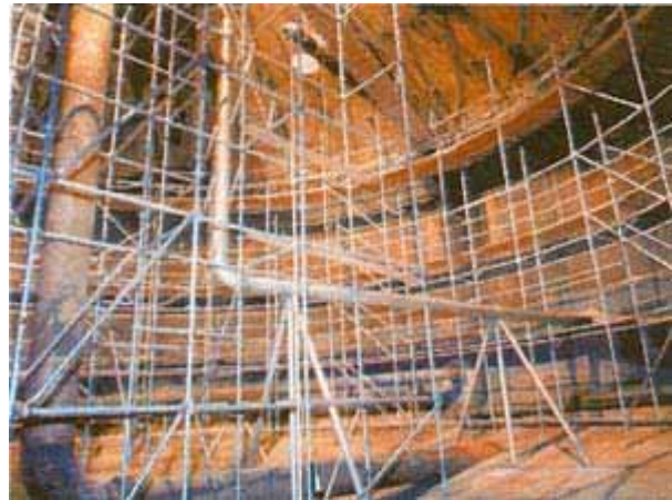
Scaffolding and Heated Sludge Return Piping Photo Courtesy of NYCDEP
