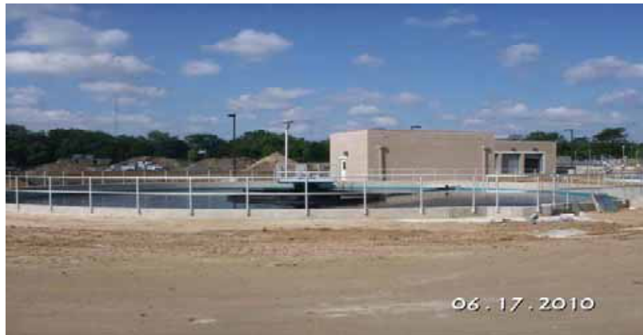
New Final Clarifier, and Return Sludge and Blower Buildings Photo Courtesy of TOMSA
