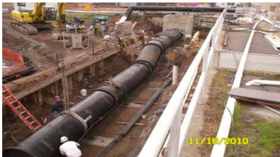
New 48-inch Effluent Line from Secondary Clarifiers to Chlorine Contact Tank Photo Courtesy of West Haven WPCP
