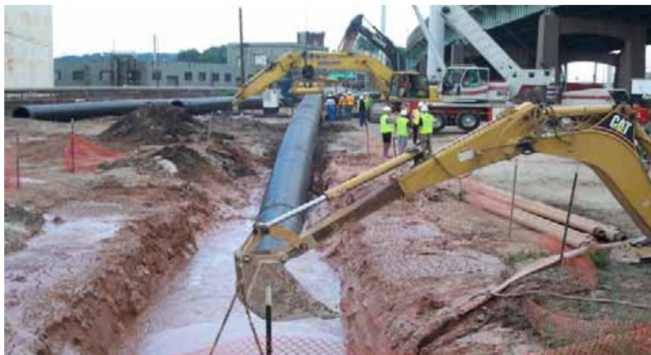
Twin 42-inch Force Mains Being Installed Beneath New Haven Harbor Photo Courtesy of GNHWPCA
