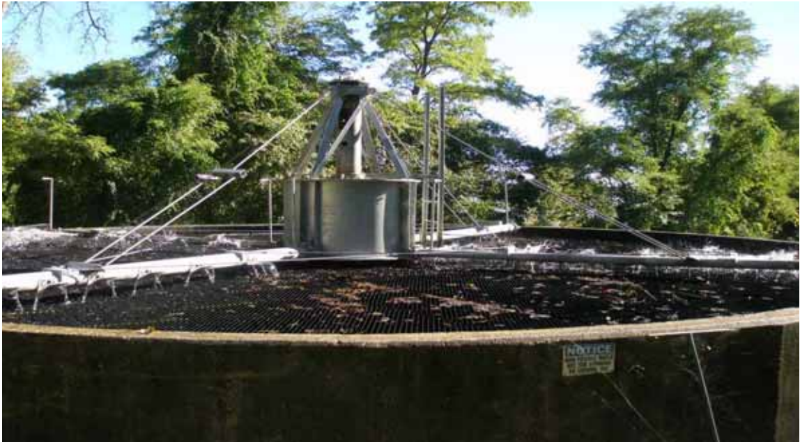
Refurbished Trickling Filter with New Distribution System and Media Photo Courtesy of R. Morlock, WWTP Supervisor, Camp Smith
