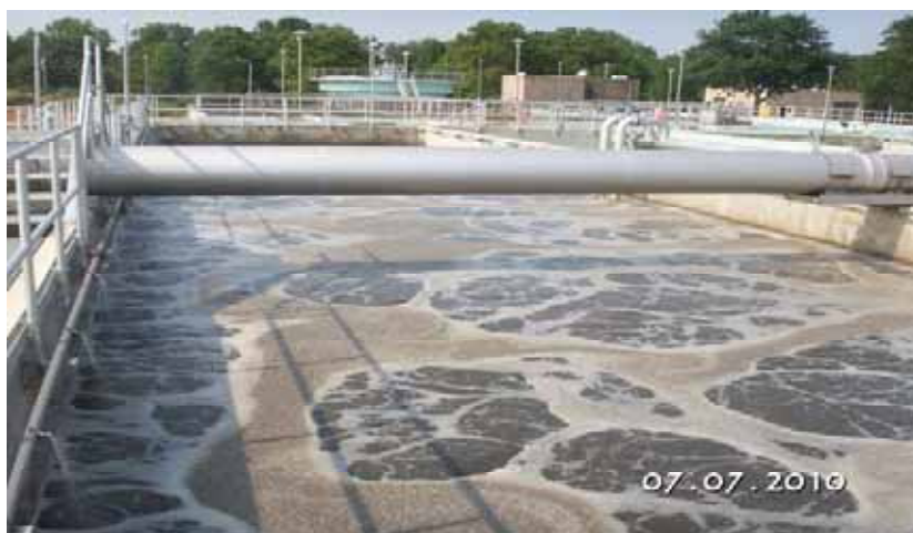
New Aeration Tanks Photo Courtesy of TOMSA
