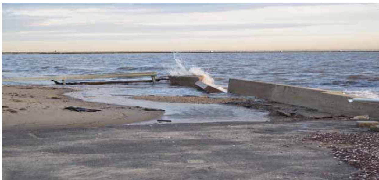
Destroyed Seawall at Leonardo, New Jersey, March 2010
