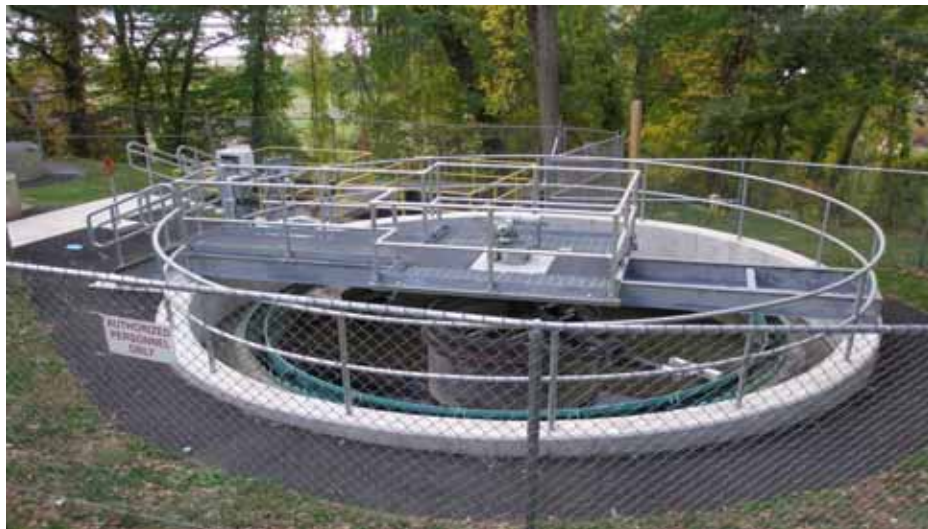
New Final Clarifier Photo Courtesy of R. Morlock, WWTP Supervisor, Camp Smith
