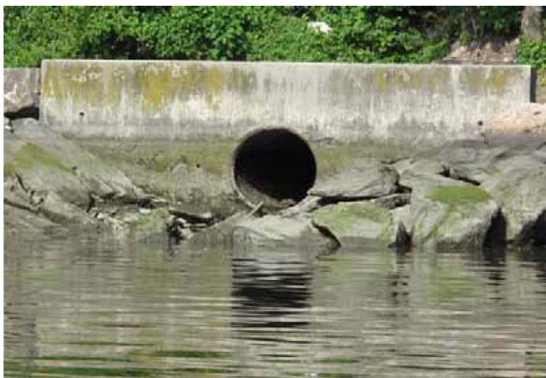
Hutchinson River Storm Outfall, June 2010 Photo by P. Sattler, IEC
