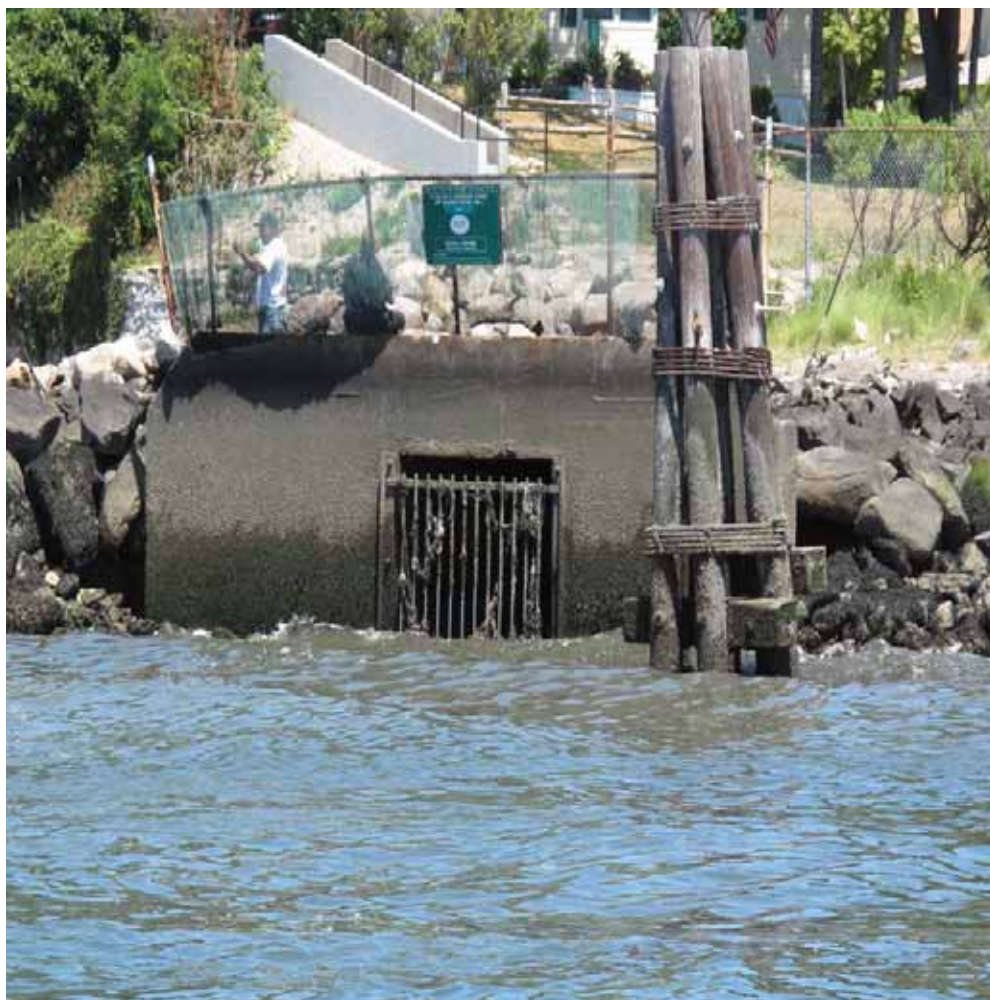
CSO Outfall on the Upper East River, July 2010 Photo by P. Sattler
