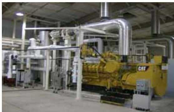
Completed Co-Generation Facility
