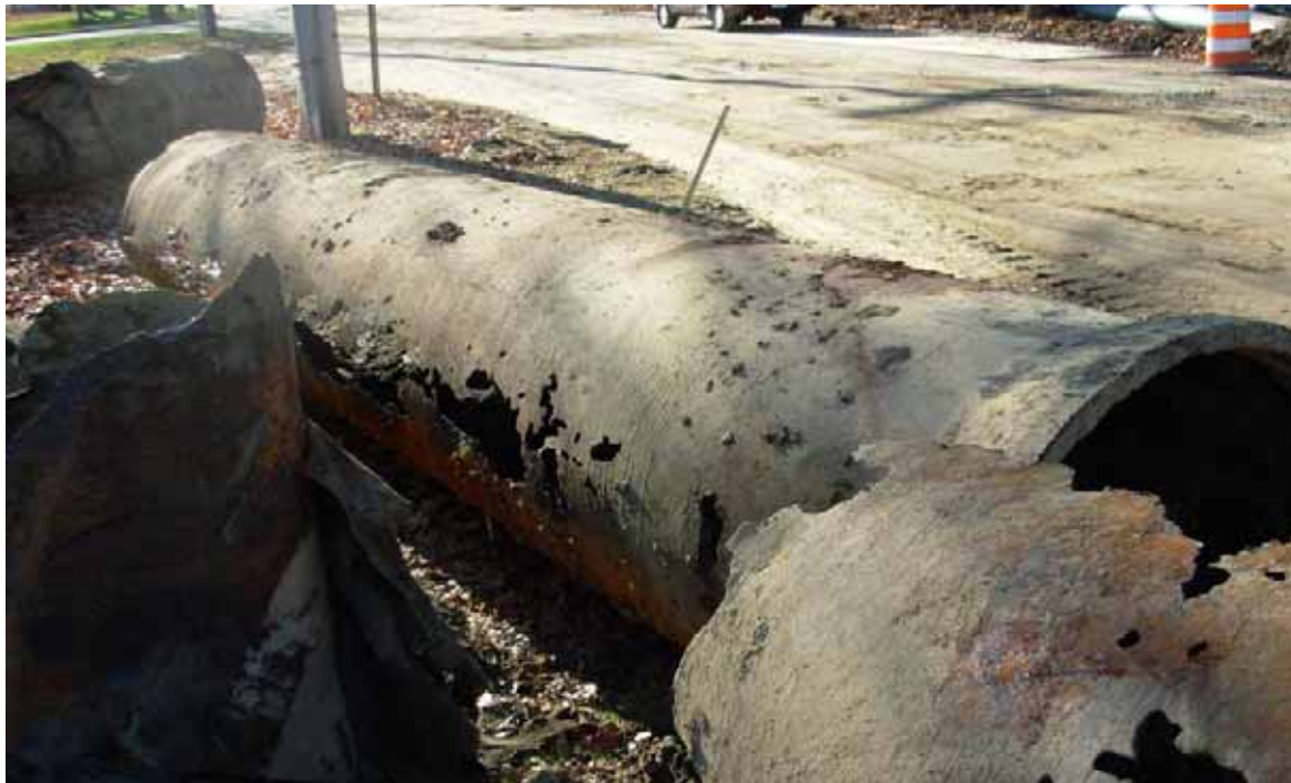
Corroded 25-year Old Ductile Iron Gravity Sewer Photo Courtesy of Milford-Housatonic WPCF
