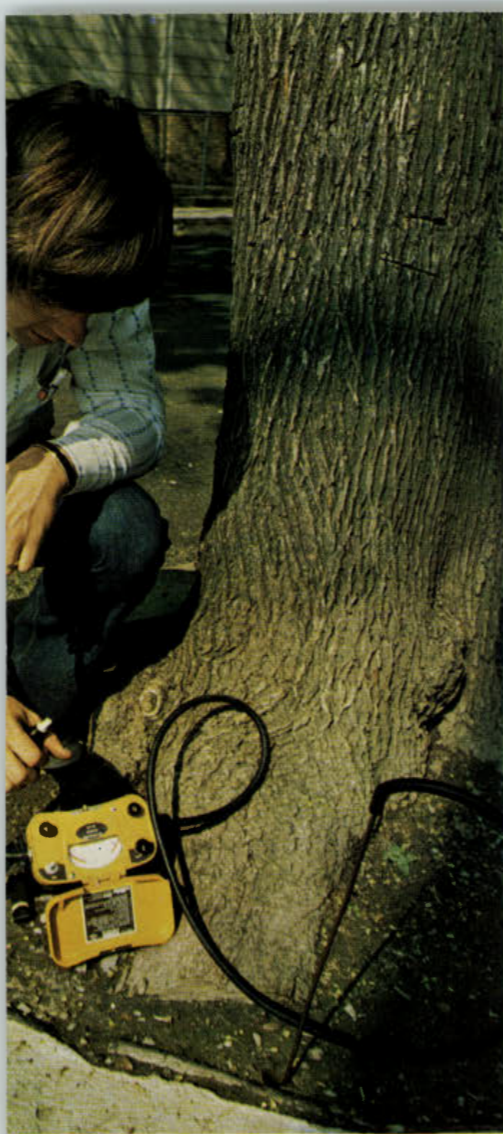
Gas probe and meter to check for tree-killing gas main leaks at base of tree.
