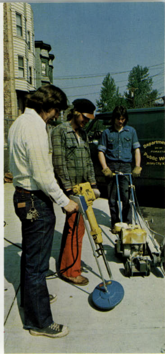
City Forester and crew using metal detector, air hammer, and concrete cutter to prepare site for a tree planting.
