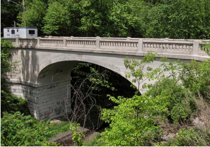
Stanhope-Sparta Road (CR 605) over DL&W New Jersey Cutoff, Byram and Hopatcong Townships, Sussex County (1911).
