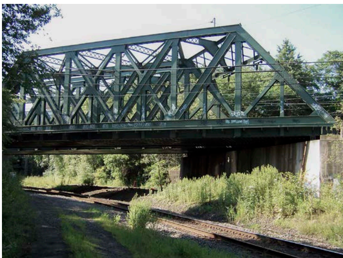
West End Through Trusses, Jersey City, Hudson County, 1908 [Source: Philip A. Hayden 2008].
