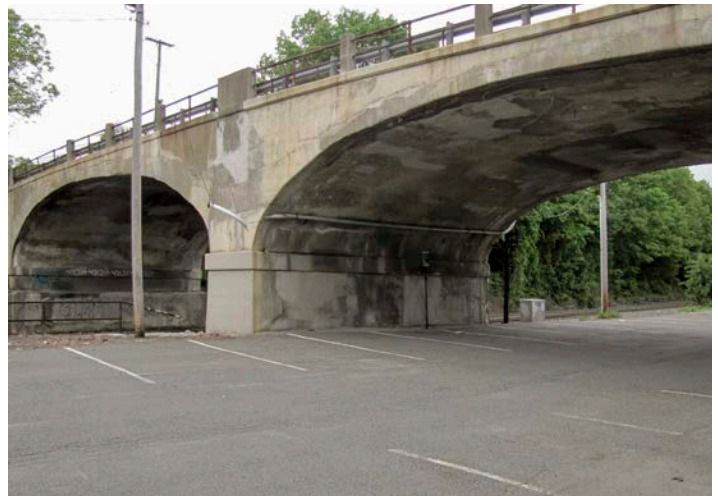
Landing Road (CR 631) over DL&W and Morris Canal in Roxbury Township, Morris County. The filled in and paved Morris Canal is in the foreground.
