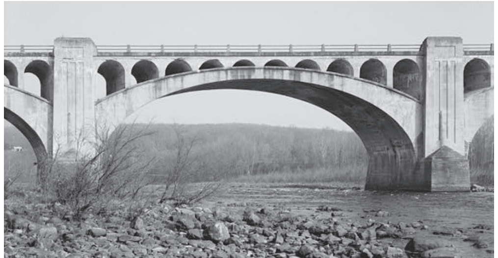
Delaware River Viaduct, Knowlton Township, Warren County, NJ and Upper Mount Bethel Township, Northampton County, PA, built 1908-11 [Source: Joseph Elliott 1999].
