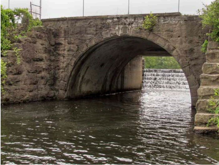
Original north face of the DL&W Bridge over Den Brook, Denville Township, Morris County (1870/1928).
