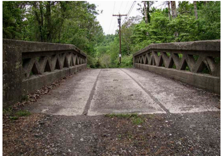
Detail of truss-like balustrades built of precast concrete on the Brickyard Road Bridge, Mansfield Township, Warren County (1913).
