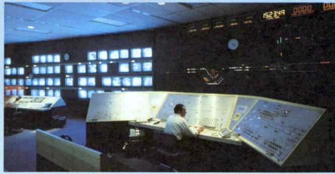
At the Journal Square Transportation Center, PATH completed and dedicated the John F. Hoban Operations Control Center, the new consolidated electronic command post named in memory of the railroad's former vice-president and general manager.
