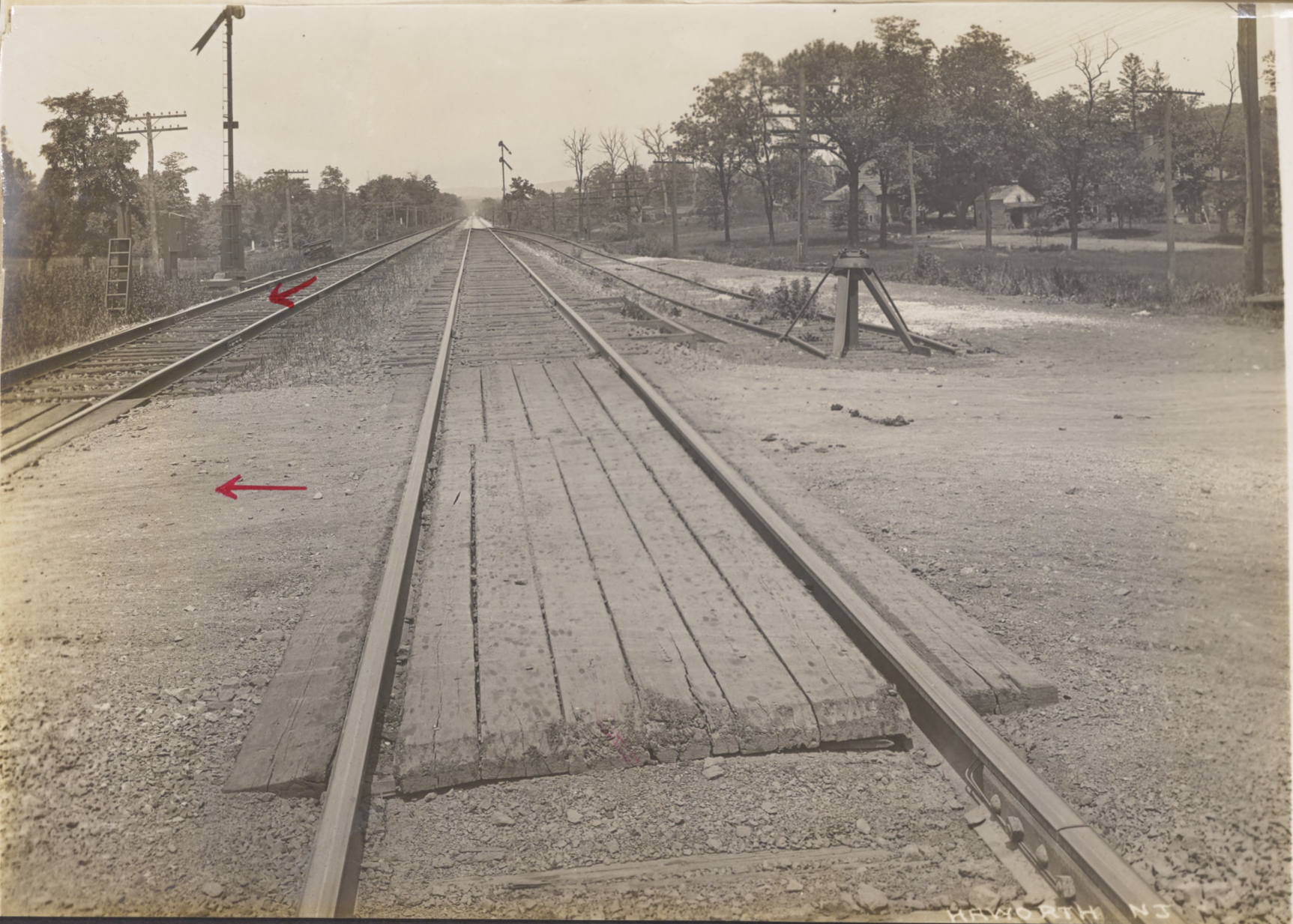
Haworth N J 4-15-15. Case, M Cattrf Plate No 4501 Detail view of crossing planks over North bound track looking North.
