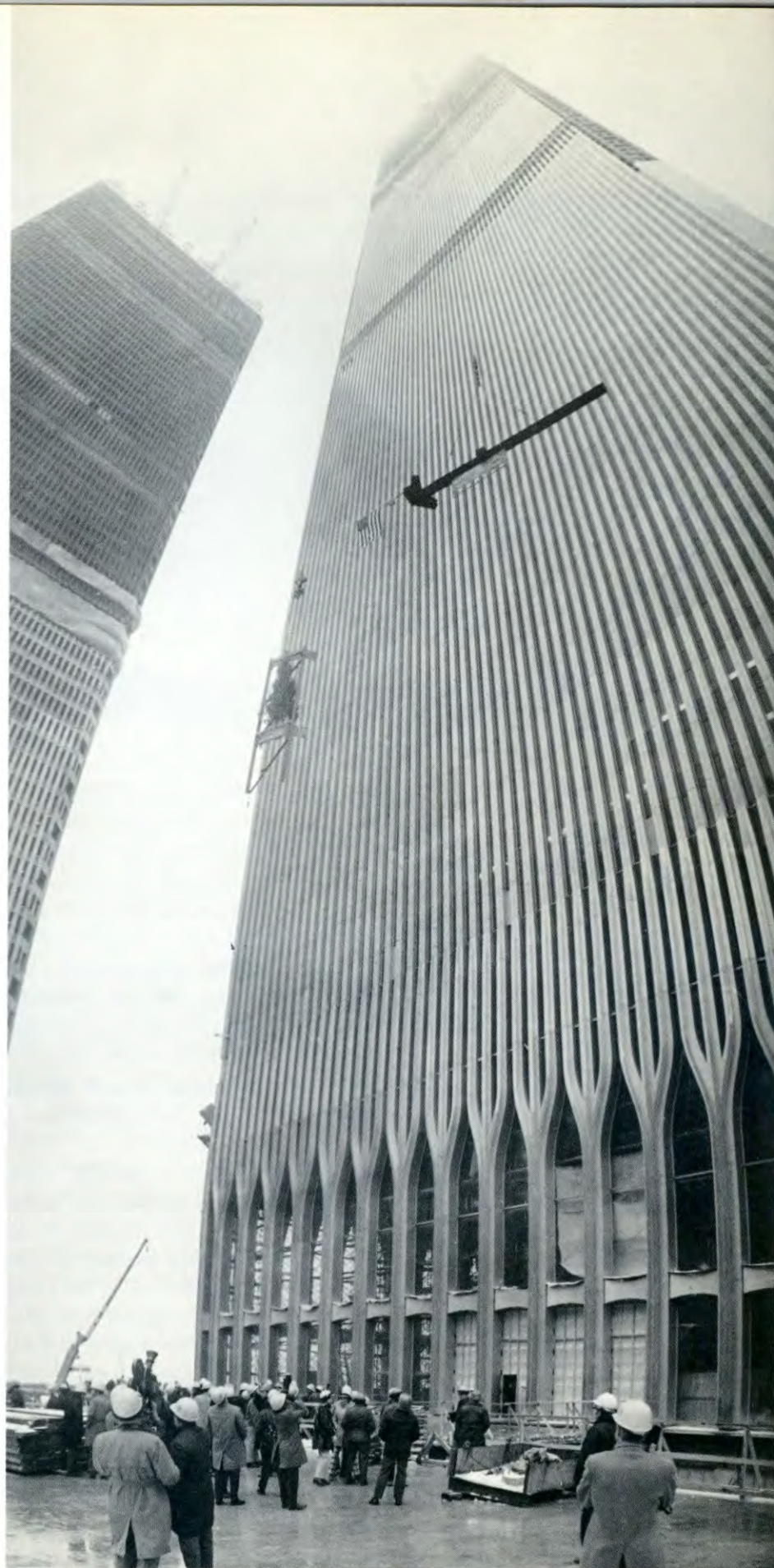
Flag-bedecked steel beam rises through swirling mist to top out the North Tower Building in December. The first tenants already were settled in their new quarters on the lower floors.
