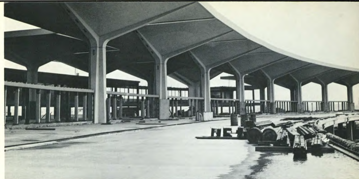
Redevelopment of Newark Airport forged ahead steadily in 1970 with the structural shell of the first concrete and glass terminal nearing completion by year's end and the airlines preparing to start interior finishing.
