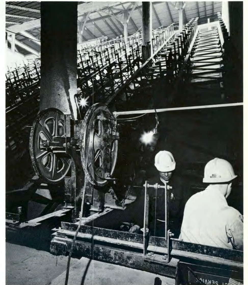
When completed, this main bank of high speed escalators being installed in the new World Trade Center Terminal will provide more convenient service to the 85,000 daily passengers using this station of the PATH mass transit system.
