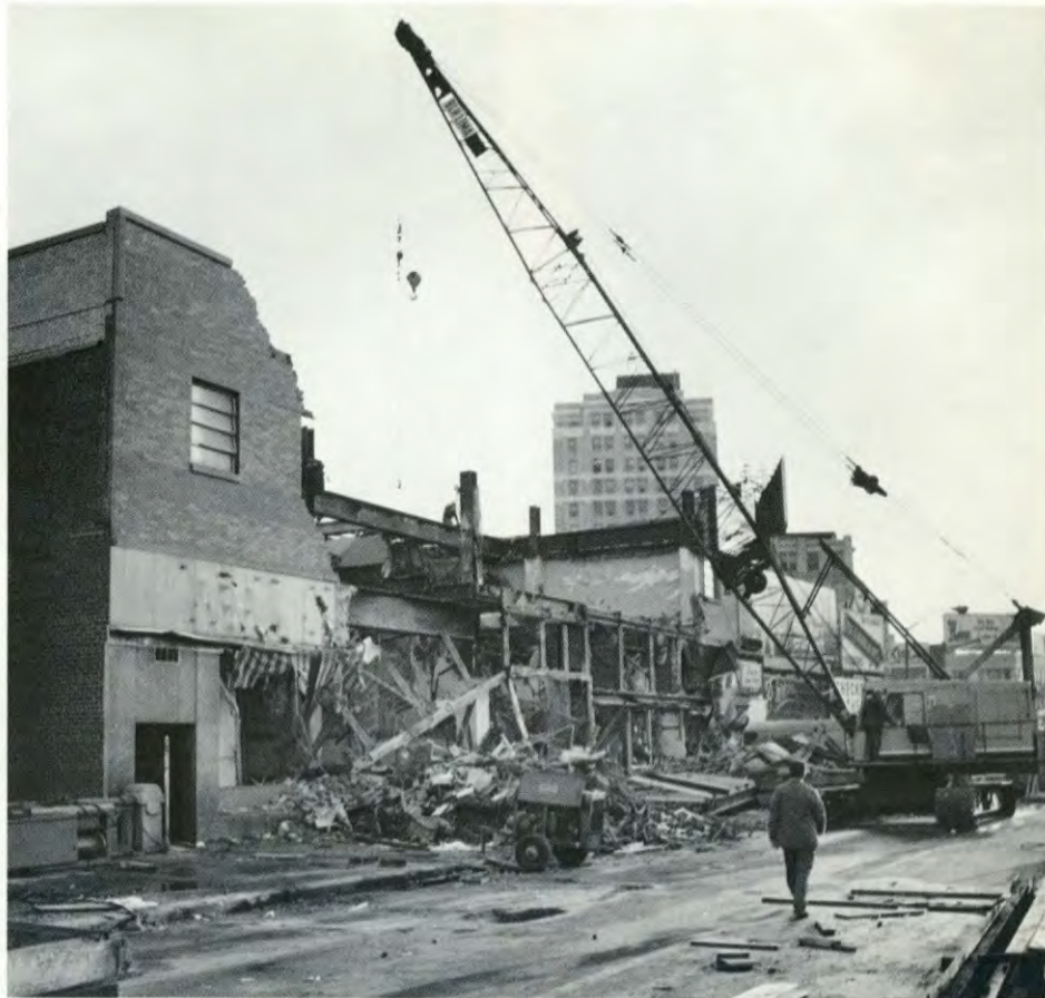
Removal of old buildings in the Journal Square area began in October to make way for construction of the transportation center scheduled for completion in 1973.
