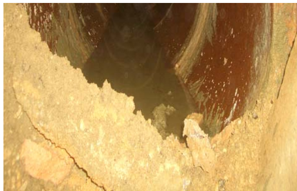
Figure 10. Damage caused to culvert by utility relocation work
