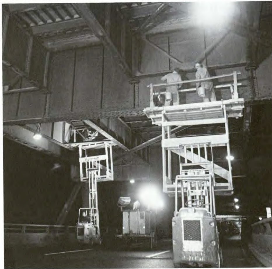
A bridge has never before been painted at night, but the George Washington Bridge finished a six-month night-time paint job on the lower level at the end of the year.
