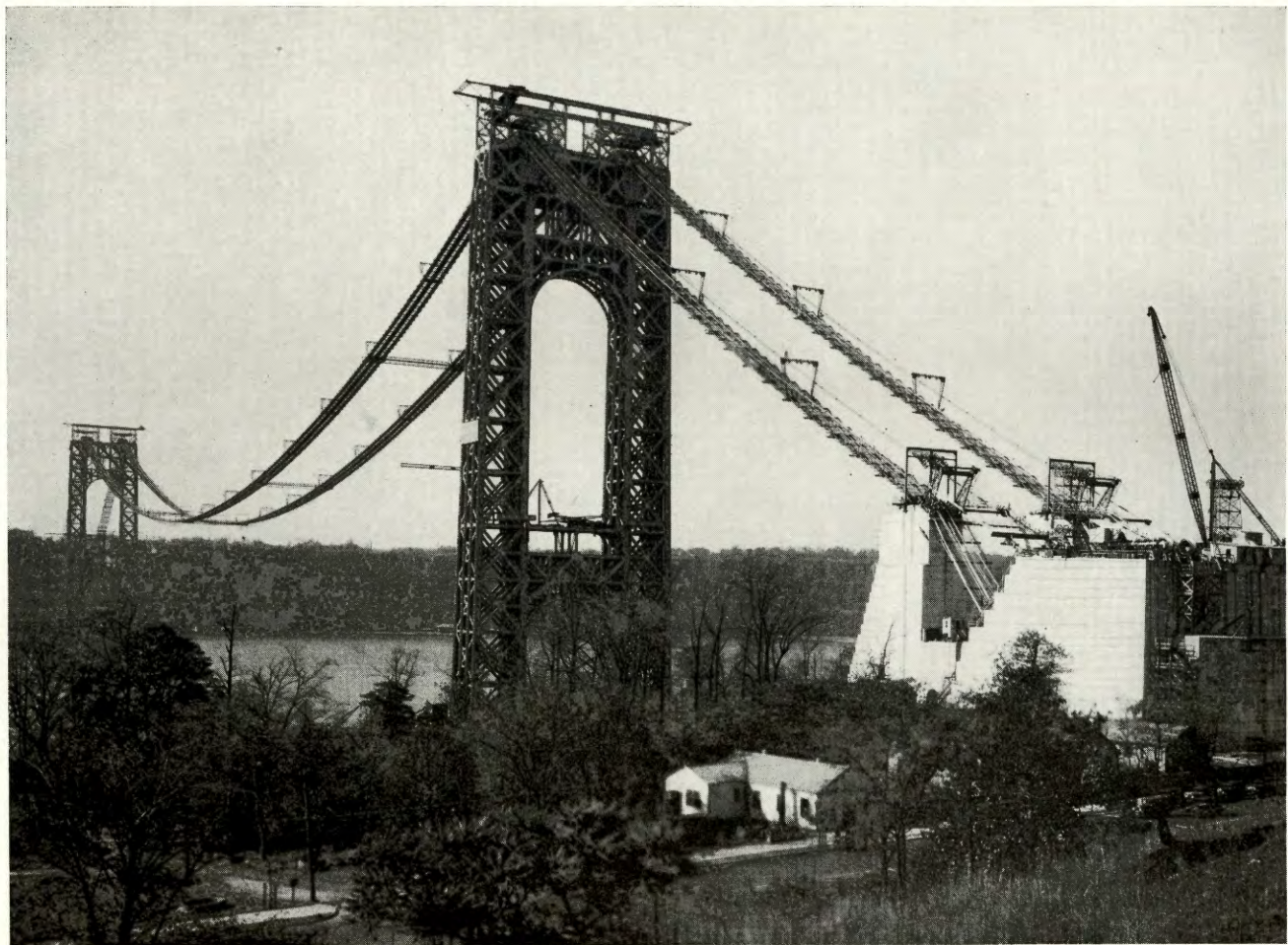
Hudson River Bridge. General View of Construction Work Showing New York Anchorage, Towers and Cable Erection
