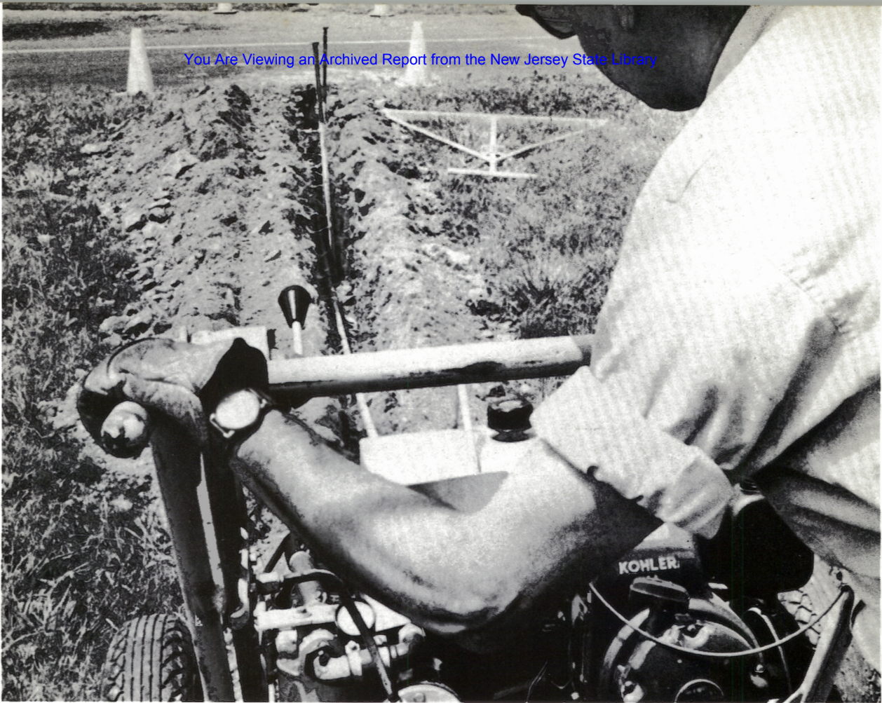
This compacting auger can bore 100-foot-long tunnels to underground telephone wires without digging up the streets and sidewalks.
