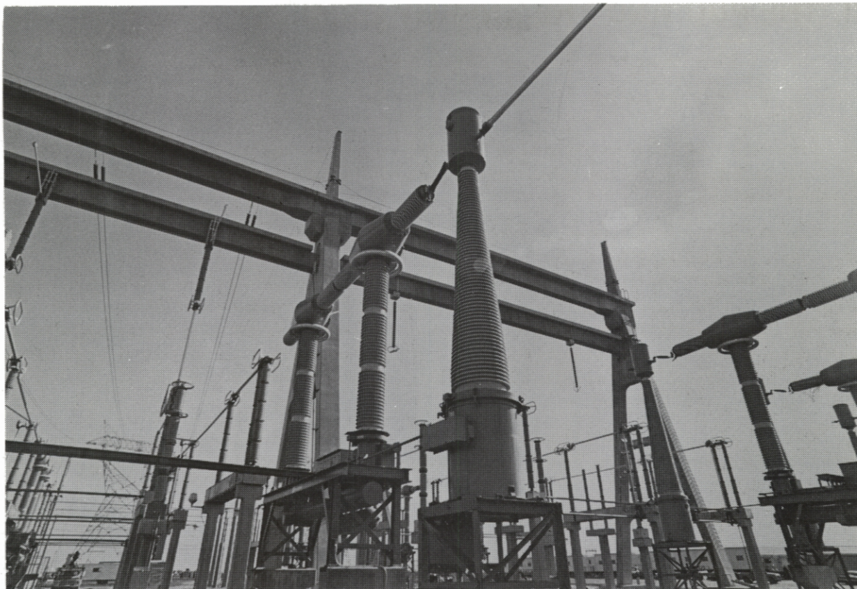
This switching station at one of New Jersey's electrical generating plants sends power through high-voltage lines (lower left) and eventually into homes and businesses.
