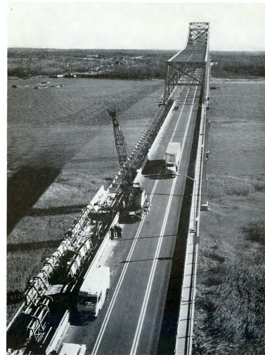
The Outerbridge Crossing between Perth Amboy and Staten Island, opened in 1928, is now undergoing rehabilitation and modernization. The improvements include the installation of modern mercury vapor lighting, the replacement of five-foot-wide strips adjacent to each curb along the entire two-mile length of the bridge, the widening of the 8,000 feet of viaduct approach roadways in New York and New Jersey from 42 feet to 50 feet to provide four 12½-foot lanes in place of the existing four 10½-foot lanes, and the building of new parapet walls in place of the existing steel bridge handrails. All work is scheduled for completion by the end of 1963.
