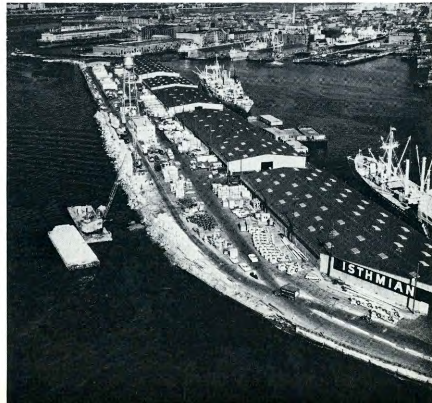
A view of the Erie Basin-Port Authority Piers showing the rehabilitation work at the outshore breakwater.
