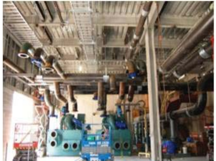
NRG Thermal's Energy Center at the new University Medical Center of Princeton at Plainsboro. The hospital is expected to open in May 2012.
