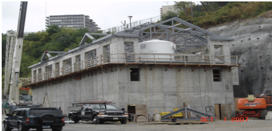
SOLIDS AND FLOATABLES CAPTURE STRUCTURE Photo Courtesy of OMI, Inc.
