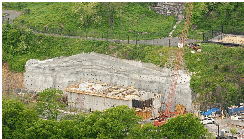
SOLIDS AND FLOATABLES CAPTURE UNIT WITH RETAINING WALL
