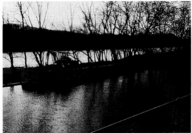
The stone wall upstream of the Wickecheoke Creek spillway was rehabilitated in the fall to repair damage caused by Hurricane Floyd in 1999.
