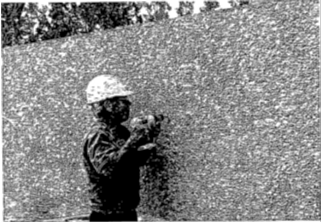
Fig 13 Grout filled plastic anchors needed tapping
