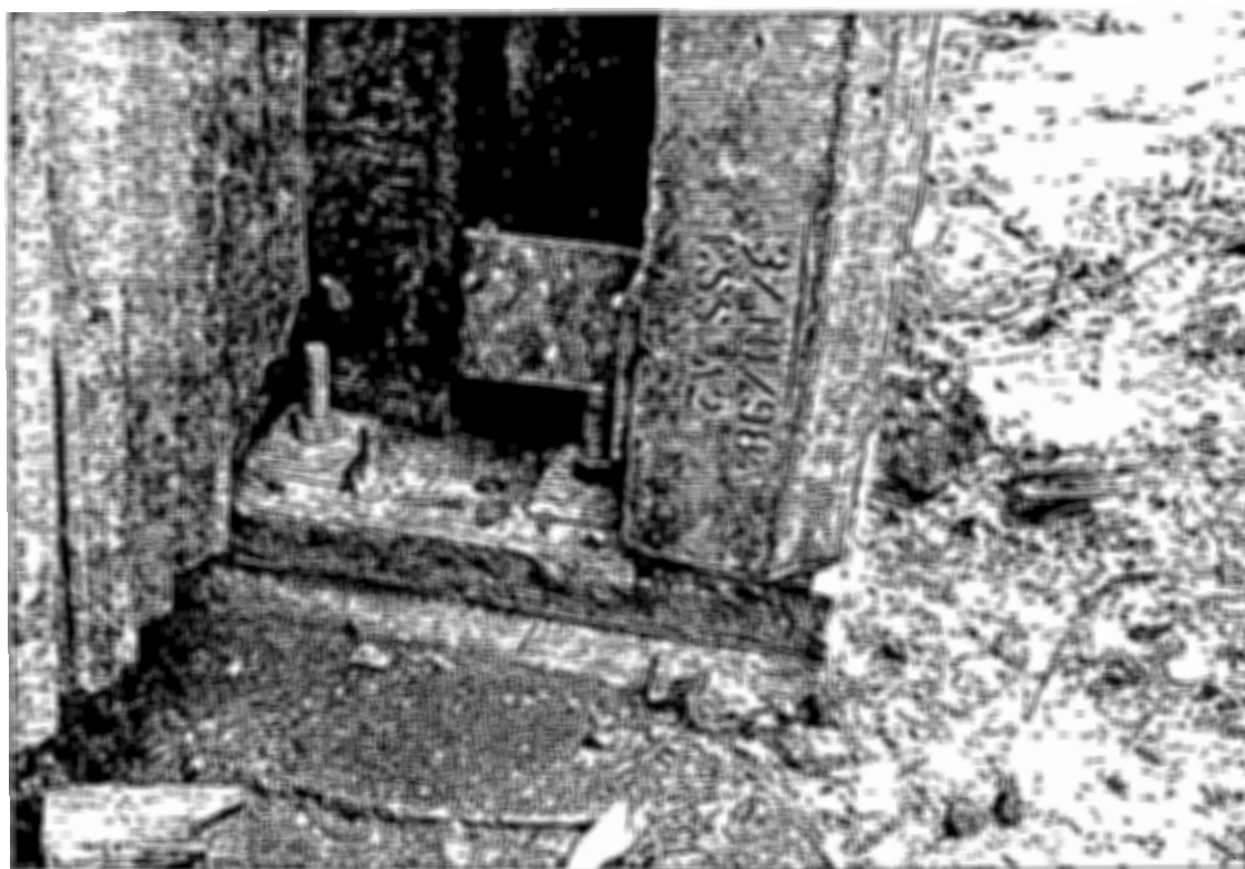
Fig 45 Post base plate set on anchor bolts with grout below Note anchor bolt and panel angle interference
