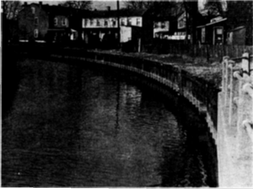
A Source of Industrial Water Delaware and Raritan Canal—Trenton Section—Sheet Steel Piling Installation
