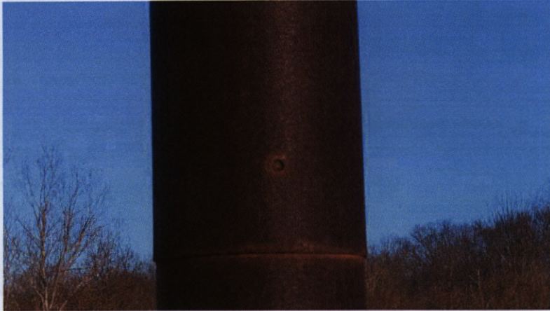
Figure 5. UAS Photograph of Potential Defect Source: NJDOT Aeronautics, 2016.
