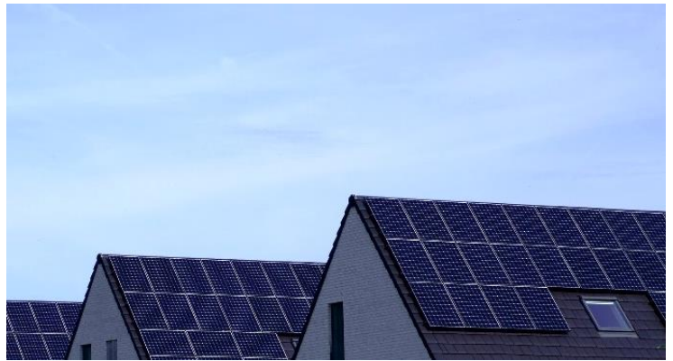
Figure 2. Example of residential rooftop solar PV.
