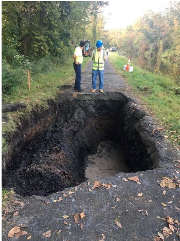
Sinkhole on the Canal multi use trail near the Workhouse Spillway
