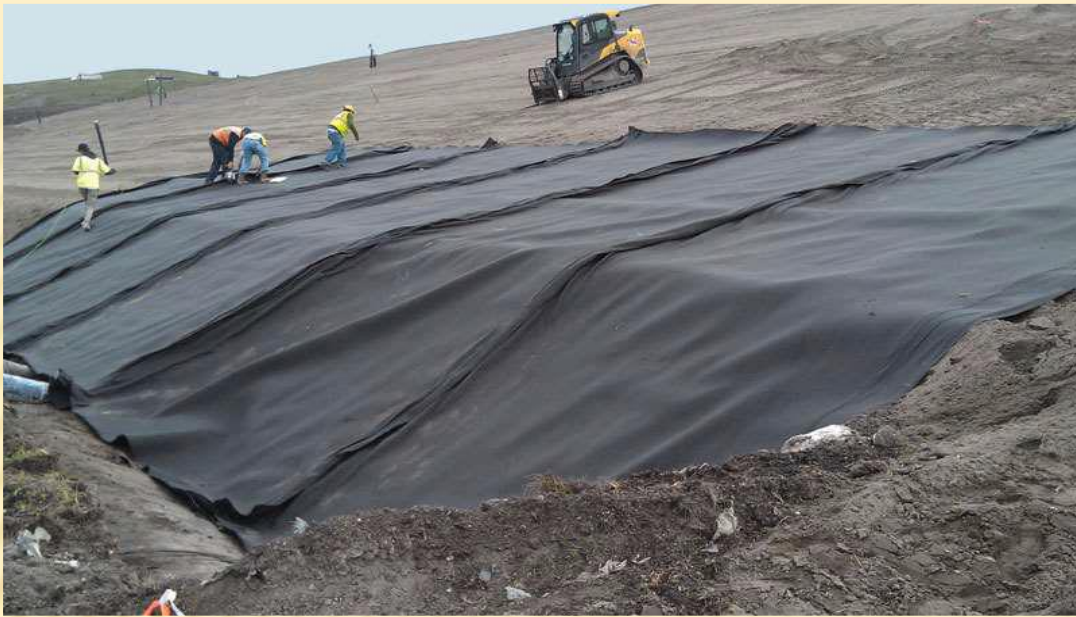
Impermeable material cap is the standard presumptive remedy ( K=1 \times 10^{-7} cm/sec) Typ. 40 mil HDPE heat or solvent welded seams
