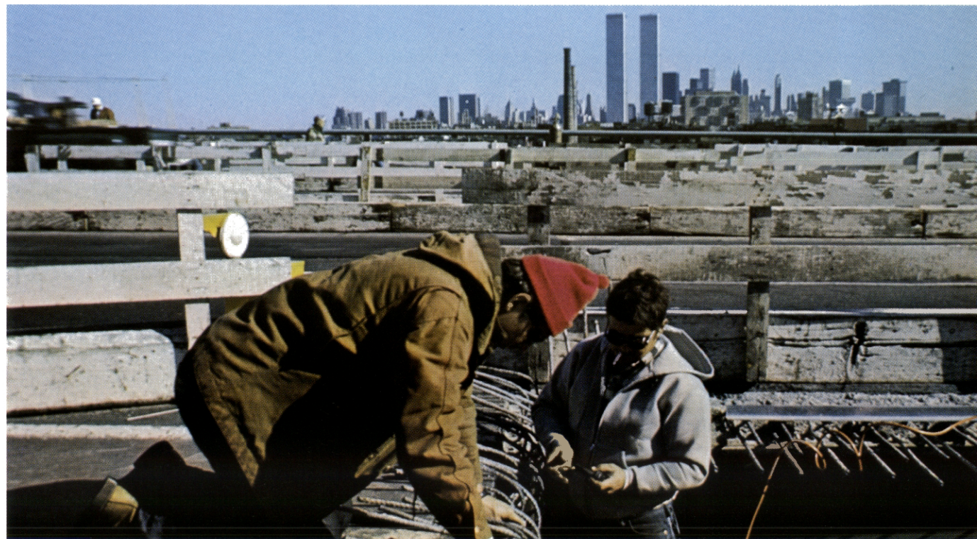
Newark Bay-Hudson County Extension undergoing major deck repairs; in the background the World Trade Center.
