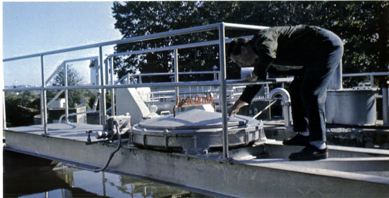
Checking of clarifier at one of five sewage plants, where the water is recycled back to earth to protect environment.
