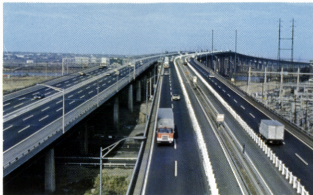
The Passaic River Bridge in early stage of widening project, during addition of shoulders for greater safety . . .
