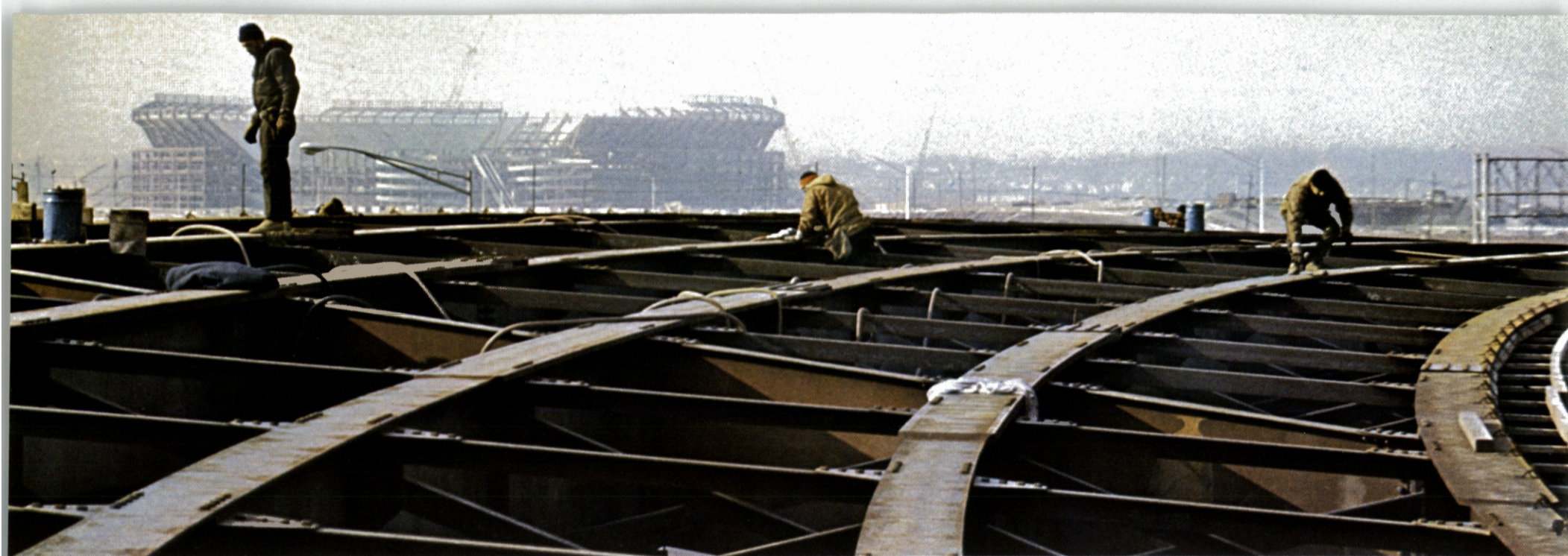
Ironworkers erecting steel girders on flyover access ramp from Interchange 18W, Carlstadt, to the Sports Complex in East Rutherford.
