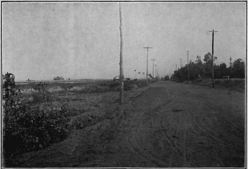
Clayton and Glassboro road, opposite gravel-bed, looking south, Gloucester County, during construction, showing sub-grade.
