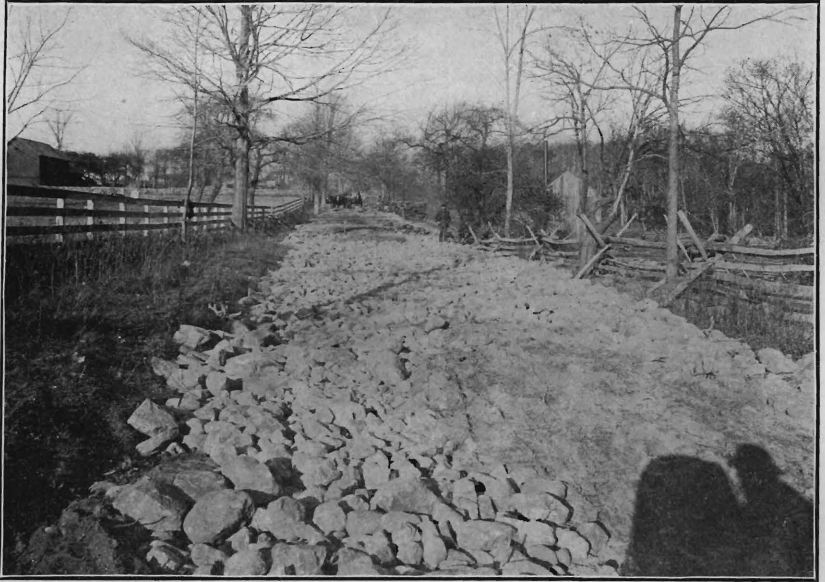
Echo Lake and West Milford road, Passaic County, northerly portion, during improvement.
