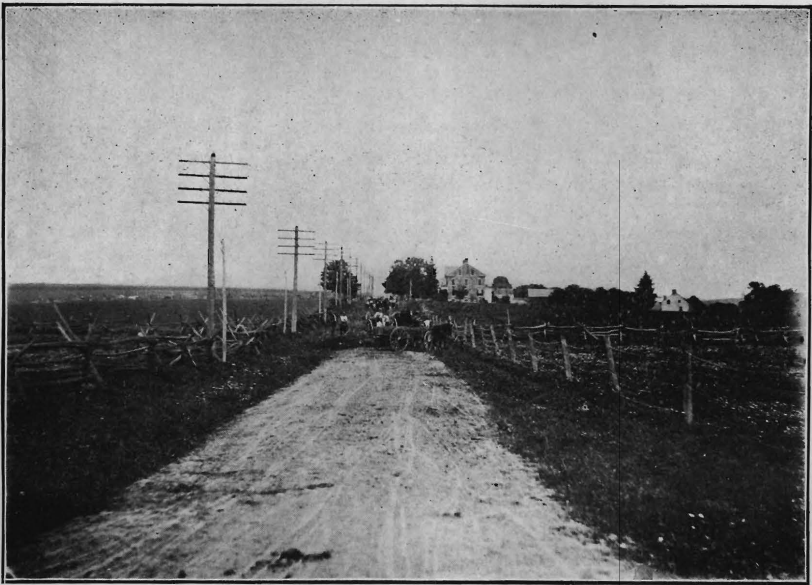
Grading Morris turnpike on east side of Pohatcong Creek, Washington, Warren County.
