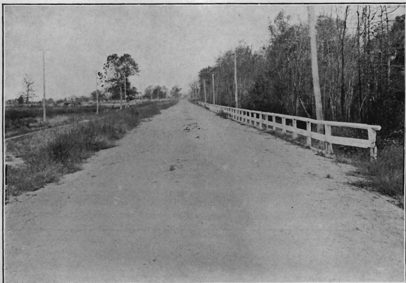
Clayton and Glassboro Gravel road, Gloucester County, opposite bog, looking north, after one year's wear.
