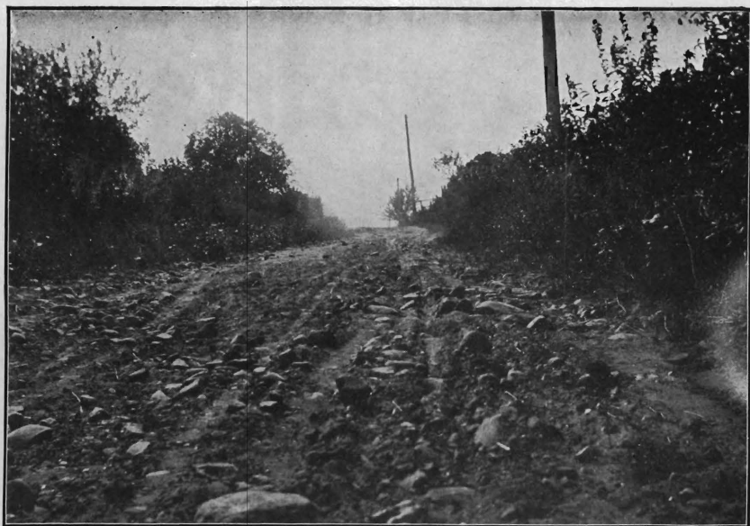
East Passaic Avenue and Kingsland road, Essex County, before improvement.
