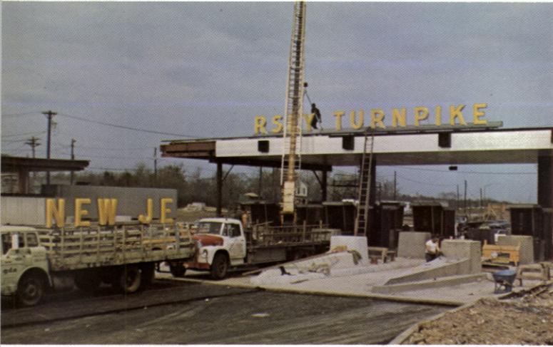
Progress is shown here as the first letters of the Turnpike name are erected at expanded Interchange 9.
