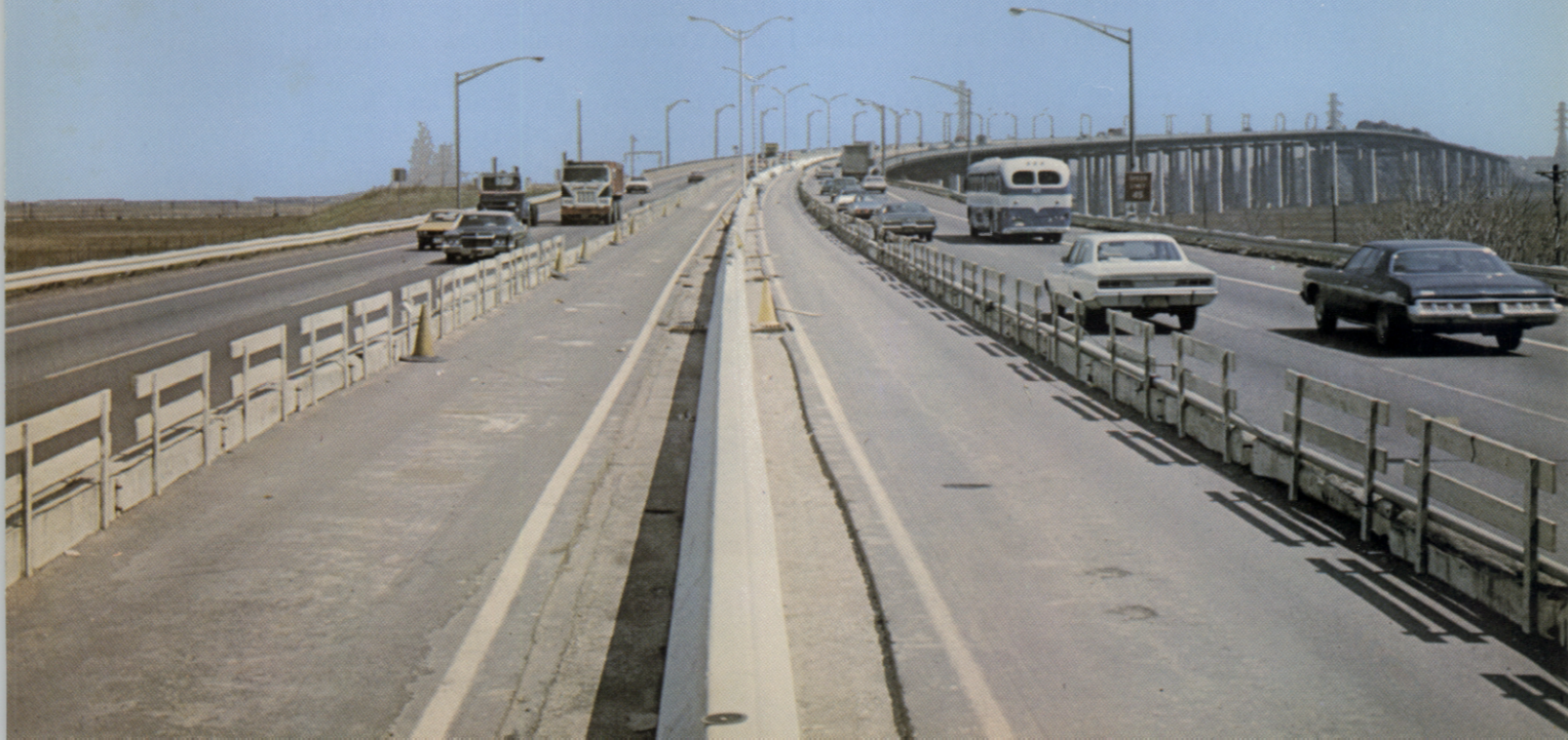
The refurbished Hackensack River Bridge shows off its new median as work progresses on expansion to include shoulders, a safety feature on all major bridges.
