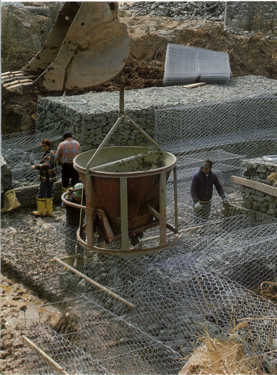
ENVIRONMENTAL PROTECTION: Fashioning a Gabion-type construction to control erosion from a wide stream along the Turnpike.
