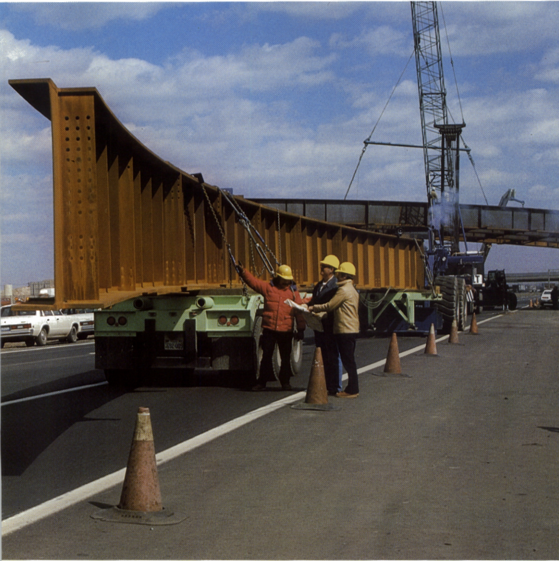
FORTY-TON steel girder rises into place for new 13A Interchange at Elizabeth nearing completion.
