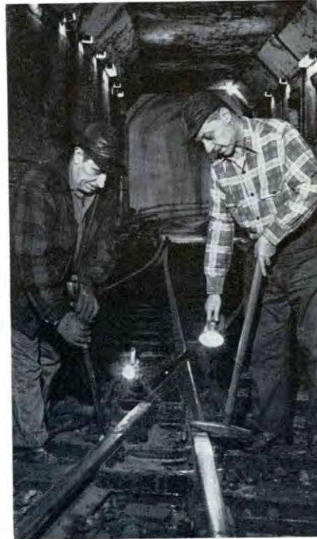
The repair and maintenance of PATH trackage is carried out without disruption of service.
