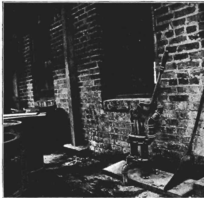
Well in Polluted Ground Beneath Building.
