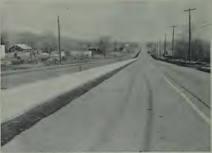
All forms being removed, the bituminous base is built up to the level of the old concrete pavement.
