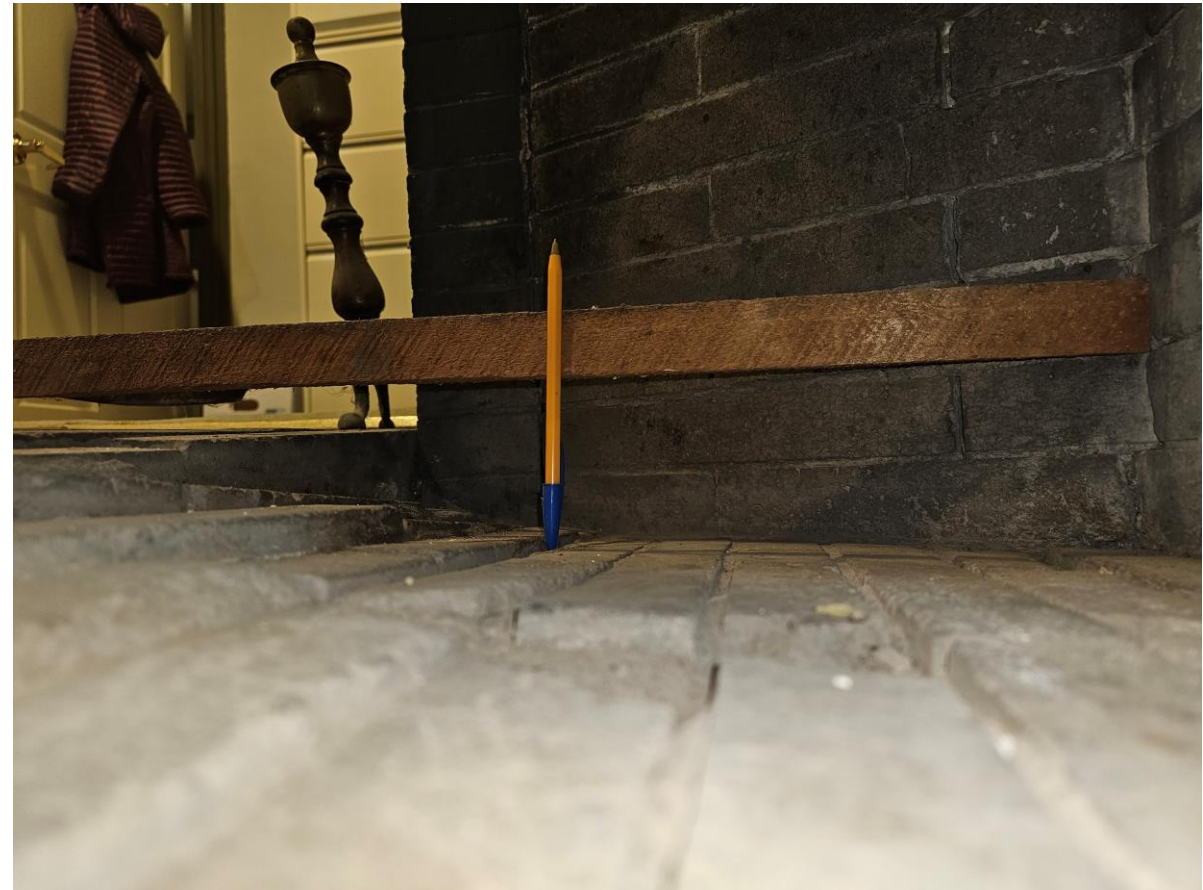
Inside fireplace showing slumping
