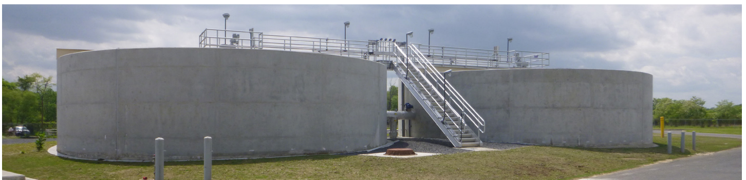
Southeast Monmouth MUA | Manasquan Water Treatment Plant Clari-Thickeners, SFY2013 Loan: $8,821,000
