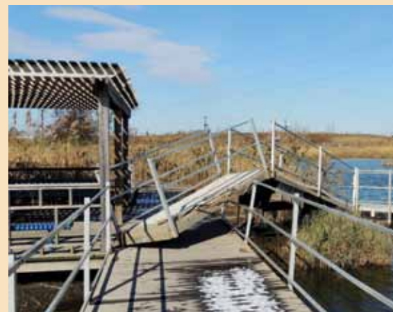
DeKorte Park Walkways damaged by Hurrican Sandy
