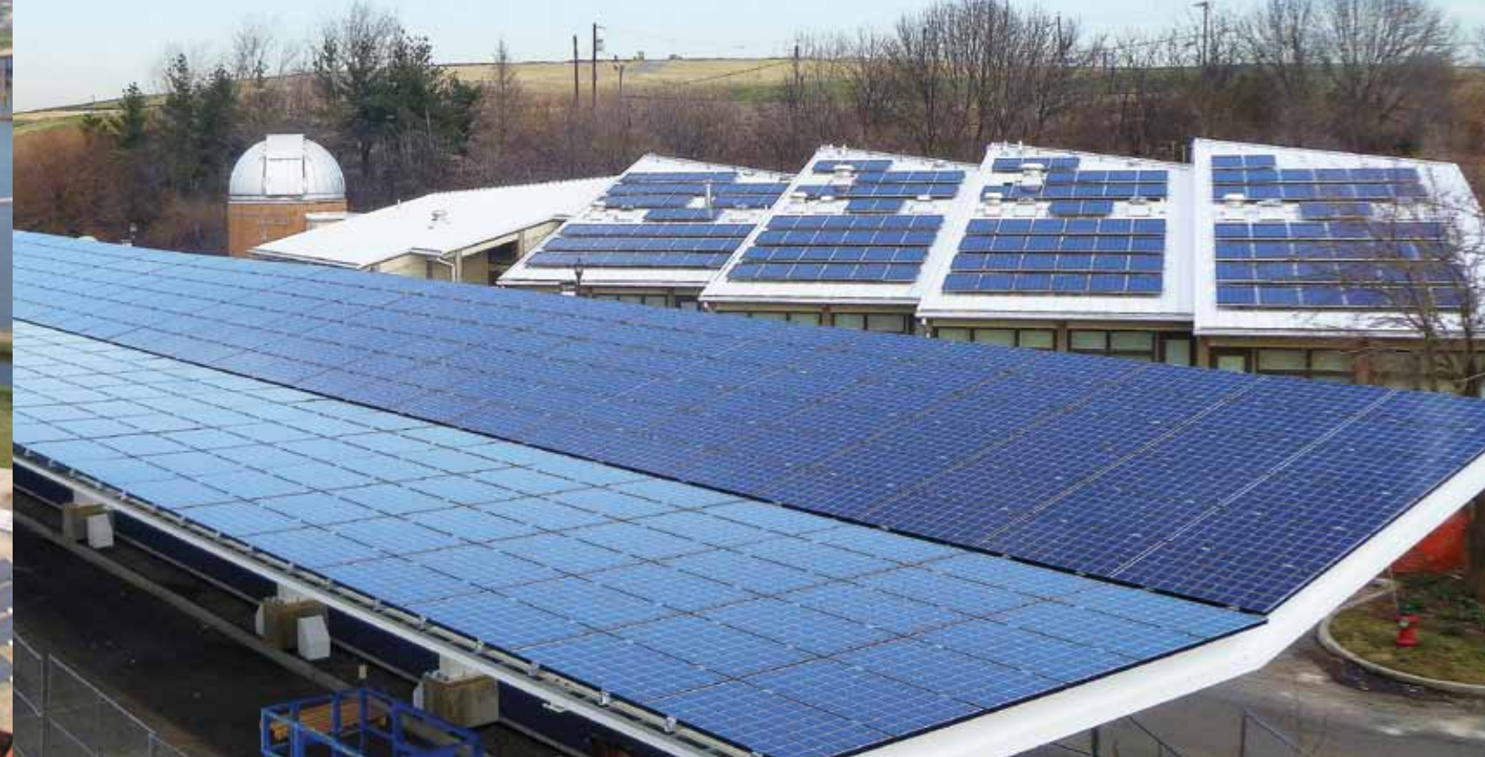
Solar Carport Canopy, NJMC Administration Office in Lyndhurst
