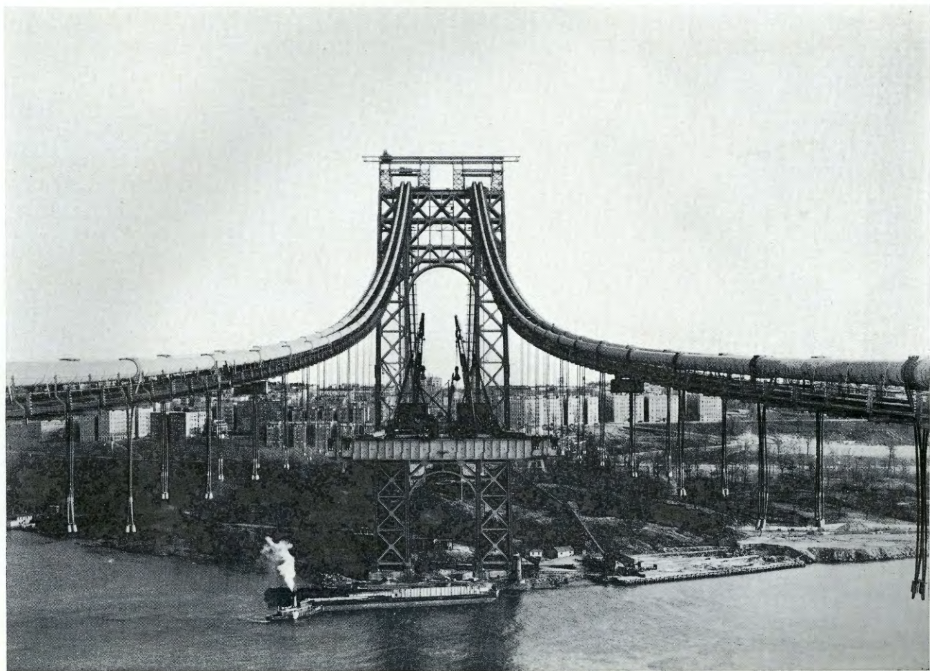
HR-1257—Floor Steel Erection near Middle of Main Span. Status of Work on December 10, 1930
