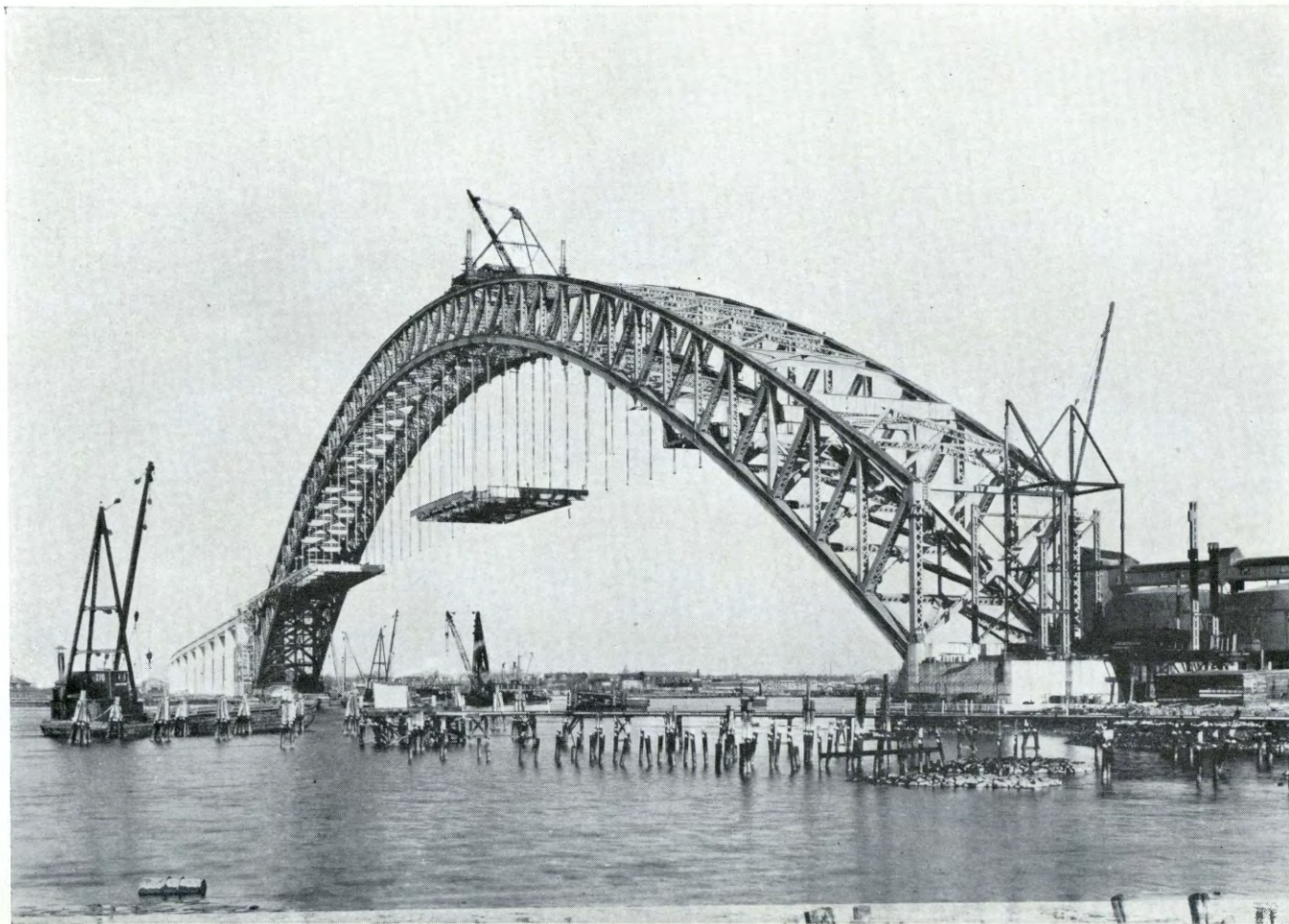
BP-599—Erecting Floor Steel on Kill Van Kull Bridge. Port Richmond Abutment in Foreground. Status of Work on December 17, 1930
