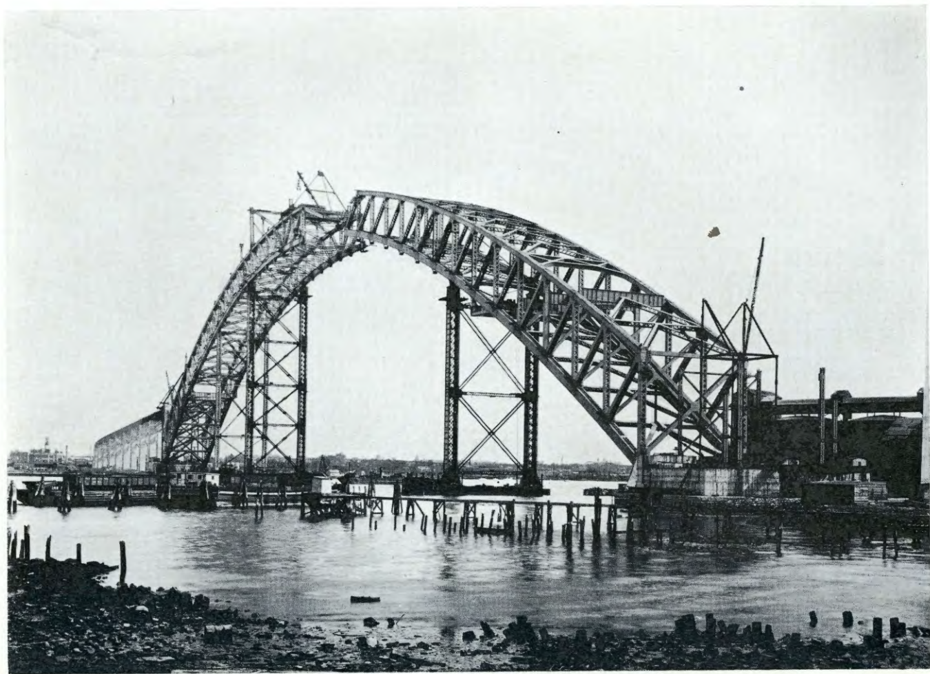
BP-571—Arch Erection Showing Falsework Supports. Traveler Working on Bayonne Section on September 18, 1930
