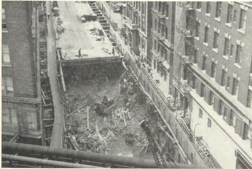
General view of progress of excavation and decking of West 179th Street Tunnel between Broadway and Fort Washington Avenue.
