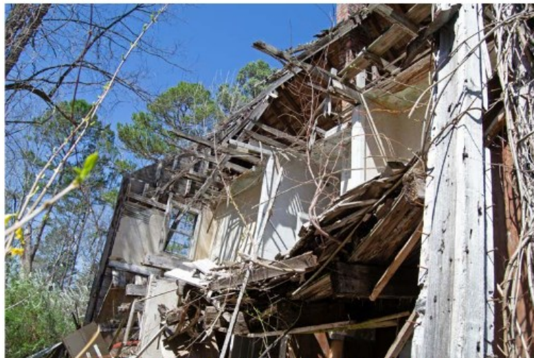
Photo 4: View of collapsed south wall, April 10, 2025.
