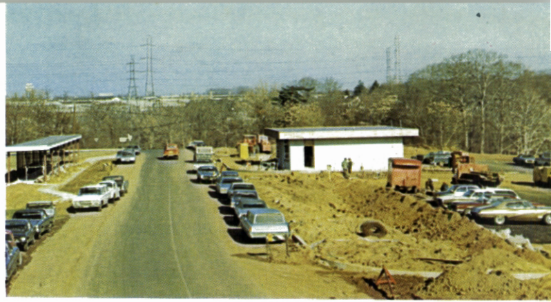
The Park-Ride in East Brunswick nearing completion. It is the Authority's first such facility to ease commuter parking congestion at site off Interchange 9.
