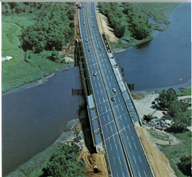
Rancocas Bridge sprouts its new 12-foot shoulders for added safety as it files across Burlington creek.
