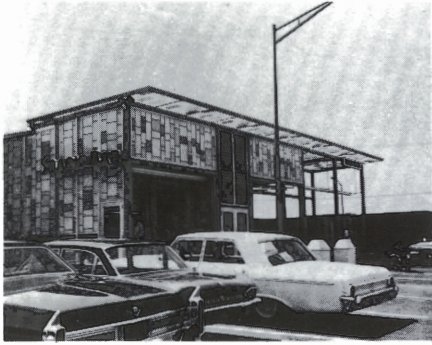
New snack bar under construction at the Thomas Edison Service Area, Woodbridge.
