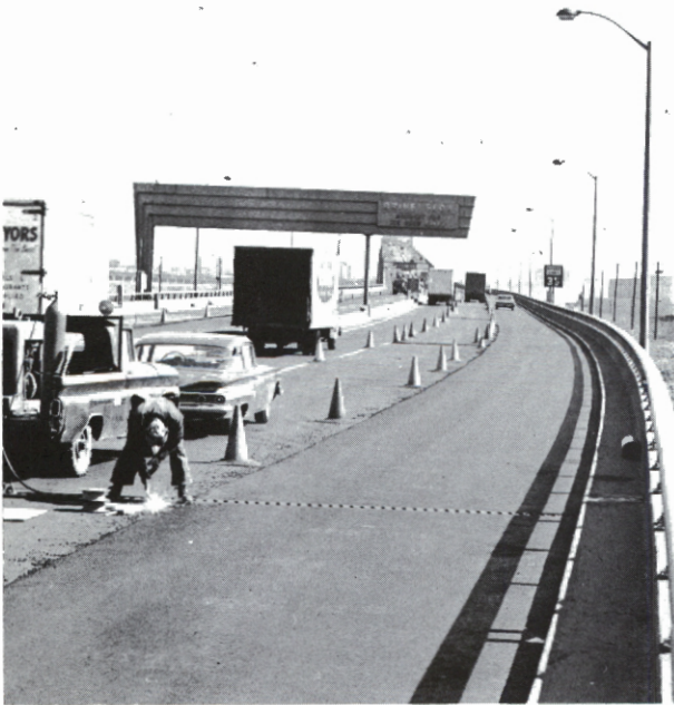
Maintenance men resurfacing lane coned off from traffic as a safety measure on the Newark Bay-Hudson County Extension.
