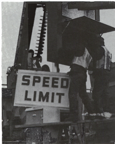
TOP: Radio tower at Moorestown Maintenance yards. CENTER: Entrance to the Turnpike at Route 46, Ridgefield Park. BOTTOM: Maintenance men installing one of many radio-controlled signs along southern end of the Turnpike.
