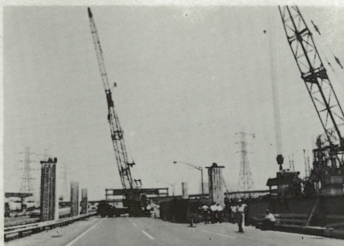
First section of steel girder being lifted into place for overhead exit ramp at the new Elizabeth Interchange 13.
