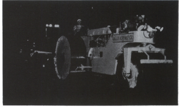
Resurfacing work goes on uninterrupted in night-time as traffic tapers off along northern section of Turnpike.
