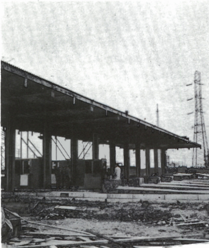
The new ten-lane toll plaza under construction at relocated Interchange 13 at Elizabeth, scheduled for completion in early 1966.
