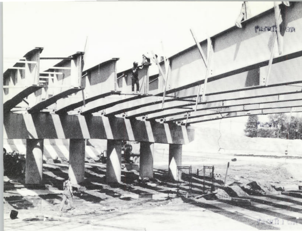
Contractors install support beams a few months before the October opening of the final, 13-mile long section of Route 55. The freeway now extends 40 miles from Maurice River Township, Cumberland County, to Route 42 in Deptford, Gloucester County.
