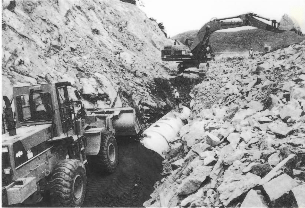
Construction crews install drain pipe along one of the last sections of I-287 in Bergen County.
