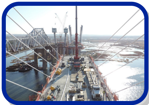
The project to replace the aged Goethals Bridge began in May of 2014.
