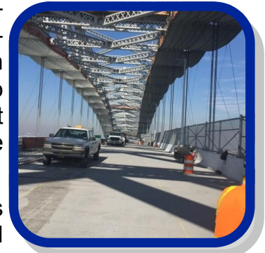
It is anticipated that the new roadways of the Bayonne Bridge will be open to traffic in February of 2017.
