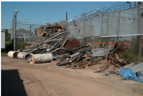
PLATE 5-26: Debris from Detention Center
