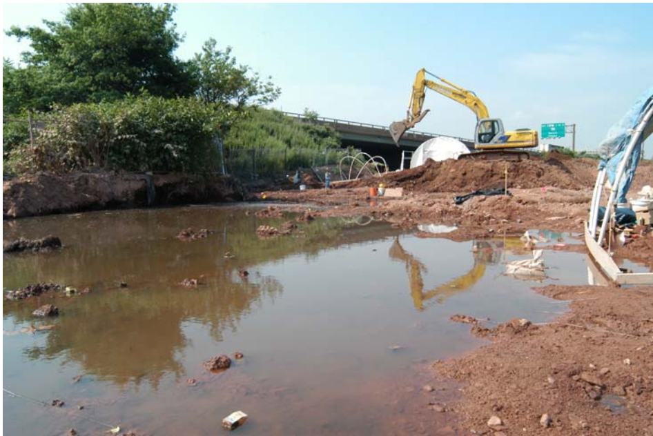
PLATES 5-18: Localized Ponding and High Water Table at Potter's Field
