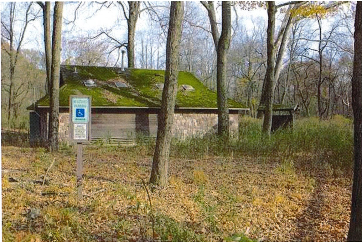
weeds grow at restroom at Bulls Island SP – it has since been demolished.
