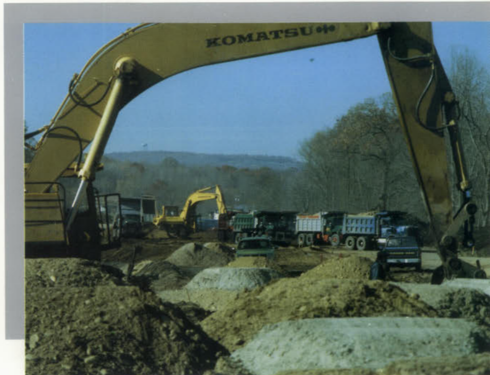
Earth movers dominate the scene on the Route 24 Freeway project in Morris County.
