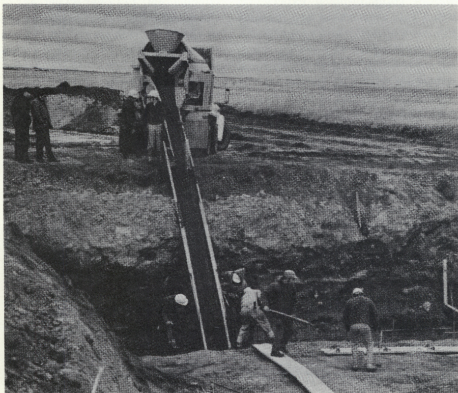
DIG . . . Workmen dig footings on what will be one of five dams on huge project in central Saskatchewan.
