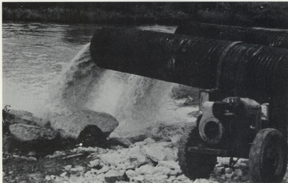
THEN FILL . . . DU dollars create another wetland area. These twin 30" pipes pour in 27,000,000 gallons of life-giving water every 24 hours.
