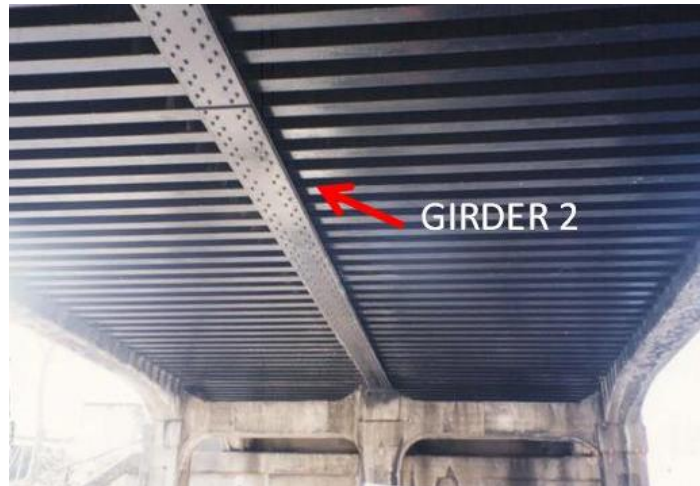
Figure 22. General view of Span 2 superstructure and underside of Girder 2 of the Main Line MP 15.95 Bridge (25)
