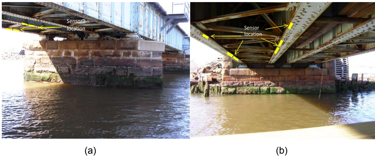
Figure 44. Elevation view (a) and bottom view (b) of a typical approach span (span length = 88 ft) of the North Jersey Coast Line MP 0.39 (River Draw) Bridge
