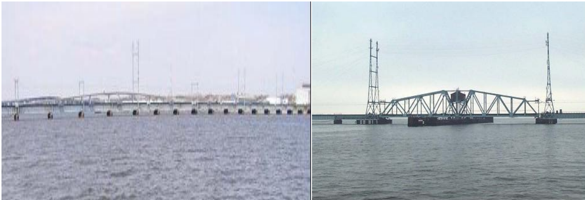
Figure 21. North elevation of east approach Span 1 to 18 of the River Draw Bridge taken from Inspection Report Cycle 4 (23)
