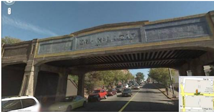
Figure 17. Elevation view of the main span and the controlling member for the load rating (center girder), view from Google Maps
