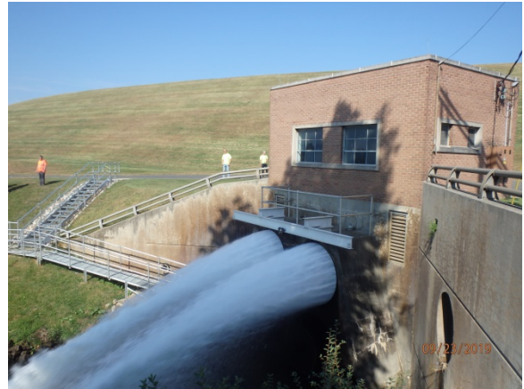
Spruce Run Vault. Howellunger Valves in Operation.
