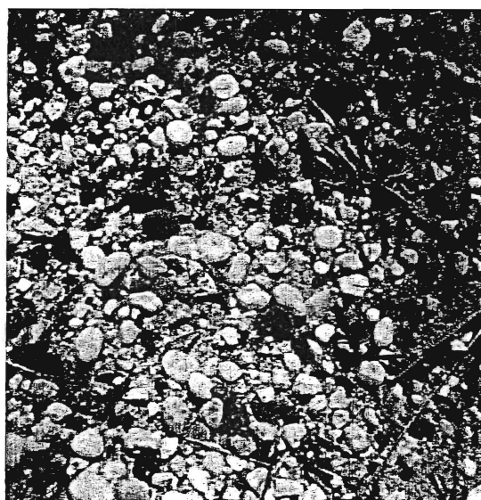
Bad non-Native Fill
