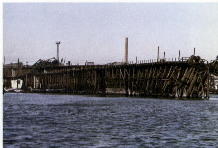
Deteriorated pier off Jersey City to be removed.
